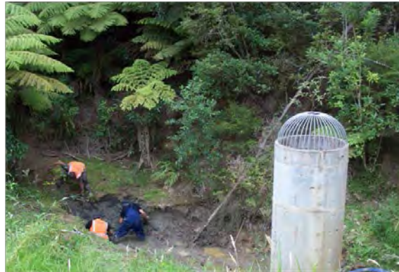
Stormwater pond being maintained by having the silt sucked out by vacuuming
