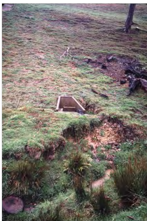
Example of erosion at a pipe outfall
