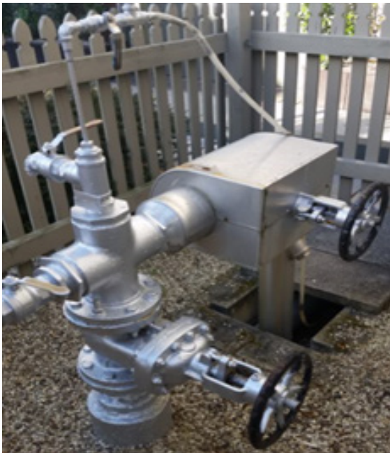
Example of a well-designed well head
