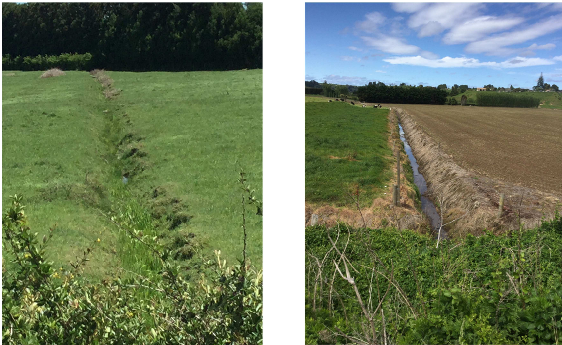
Figure 9 Examples of two small lateral drains that are common throughout the Kaituna and Rangitaiki Plains. Such drains are either generally ephemeral (left) or perennial (right), and are often either unfenced (left), or fenced with minimal setback to maximise the area of arable or pasture land.
