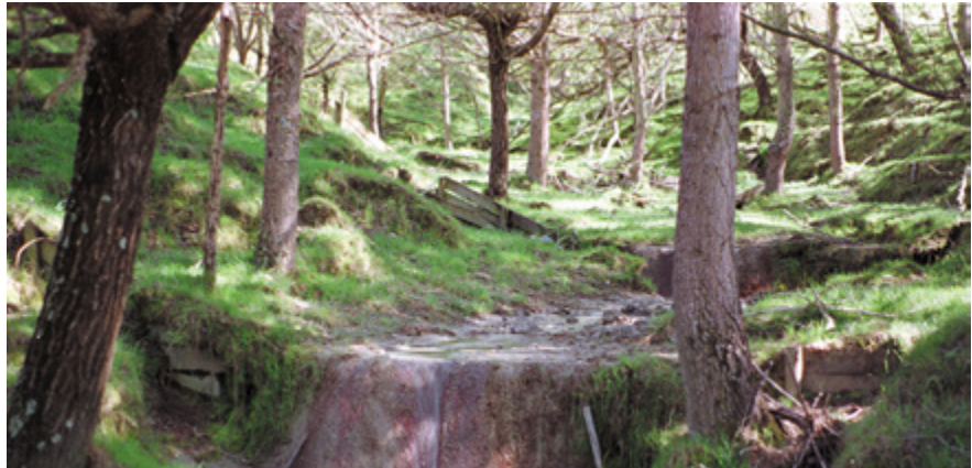
Bioengineering using willows as part of gully control works. The extensive root system provides ongoing soil stabilisation to control headward gully erosion in conjunction with check dams.
