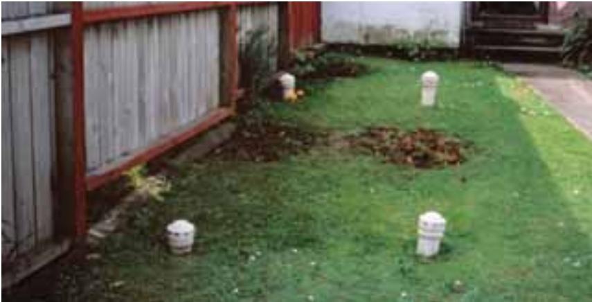
Mushroom vents above septic tank.
