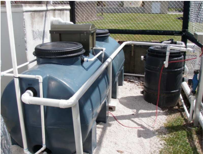
Figure 3: AWTS-N1 Treatment Tanks
