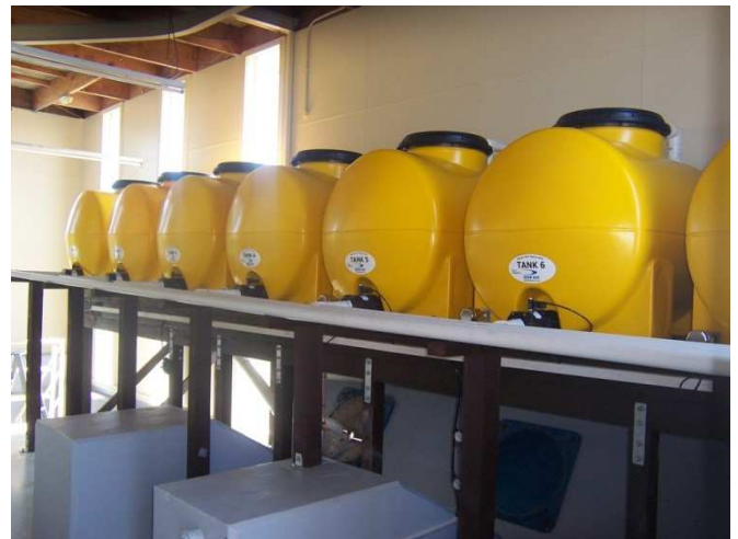
Figure 2: Header tanks delivering wastewater
